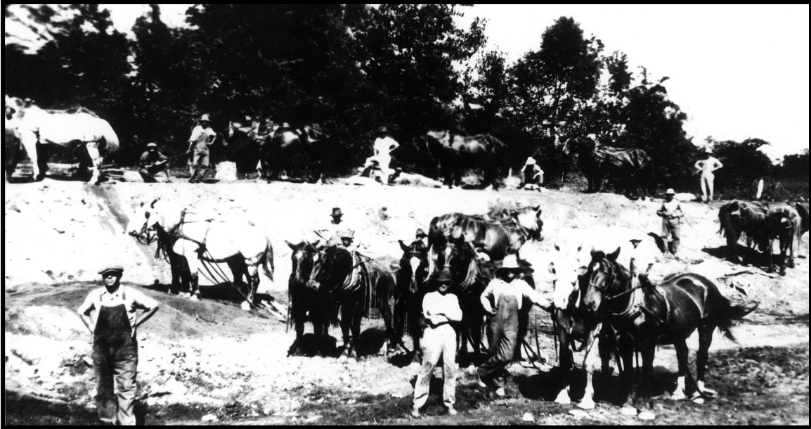
40 men using horse-drawn slip scoops dug the millrace channel at a cost of $100,000.
